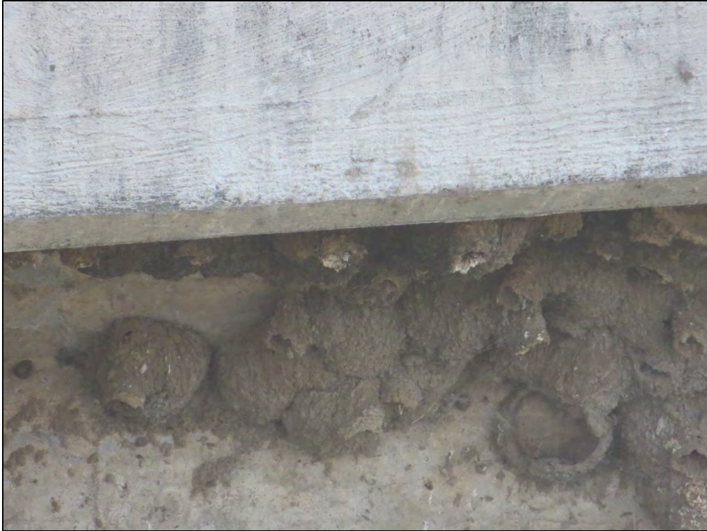
Figure 13. Swallow nests under bridge, upstream side of bridge
